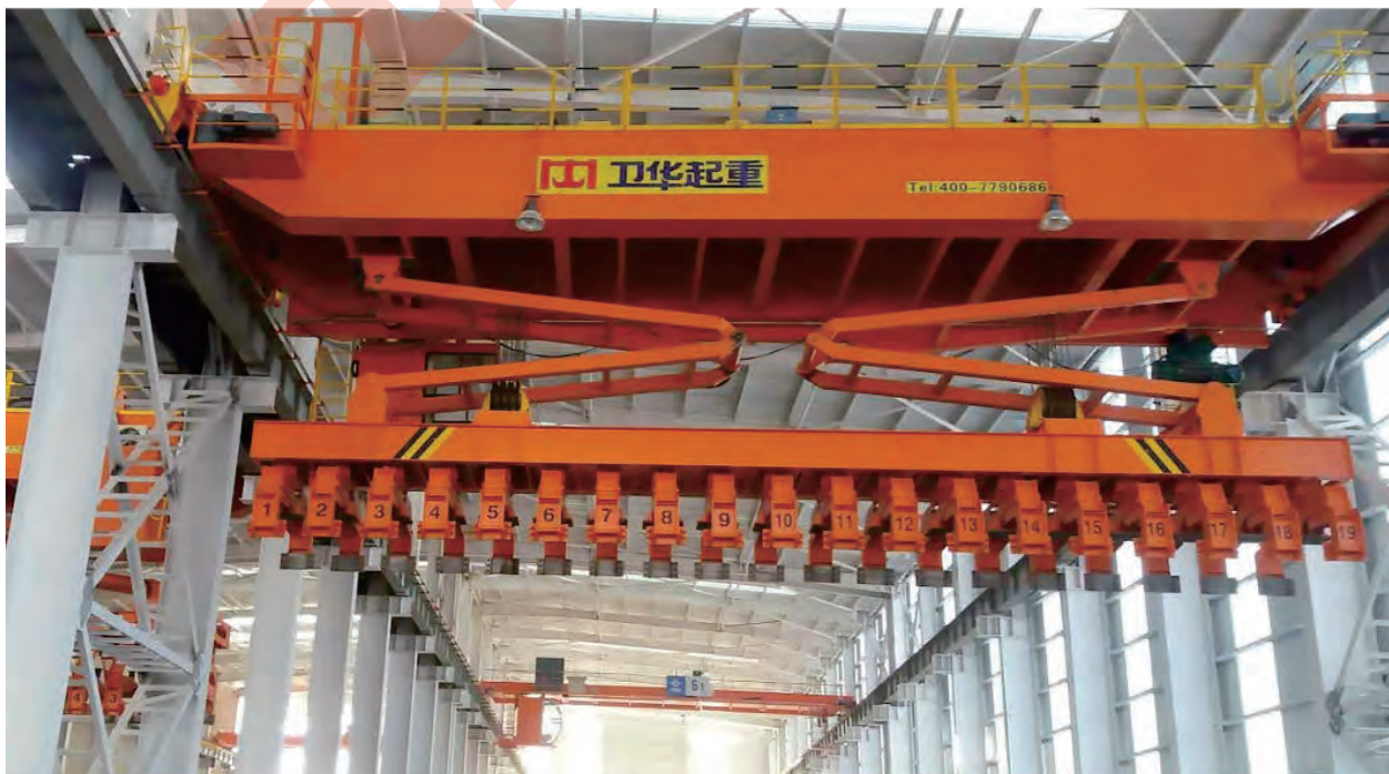
阳极炭块堆垛起重机 Anode Block Stacking Crane
